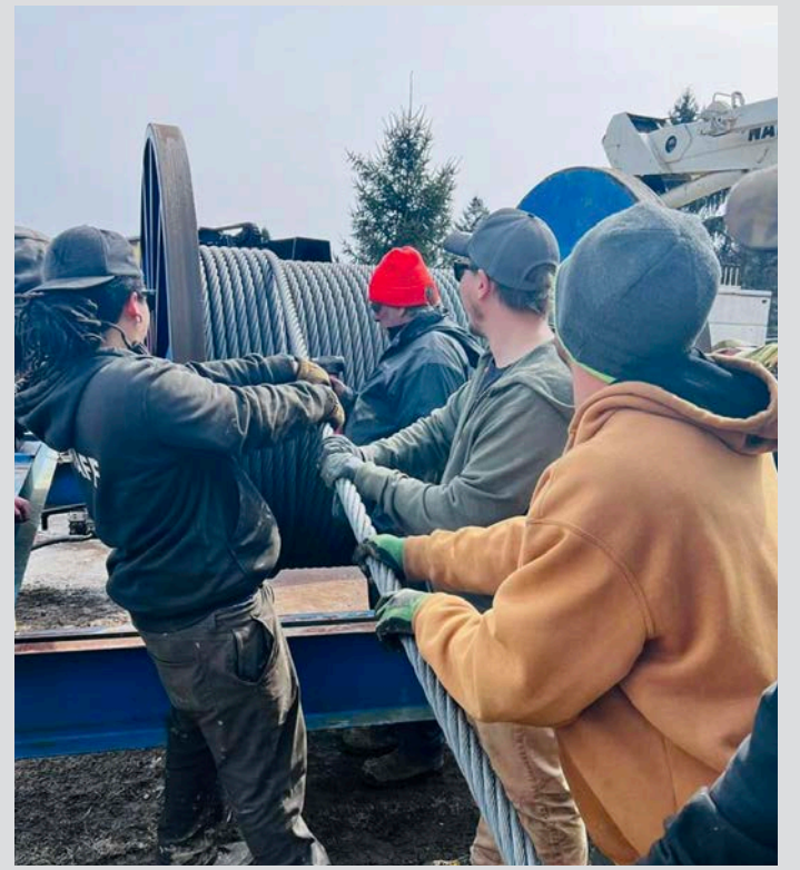
Cjcurtis1478: Well, that's a wrap. 9000ft of 42mm cable rolled up, over 40,000lbs. Great job guys! #evlnow #workinghard #rollwithit
